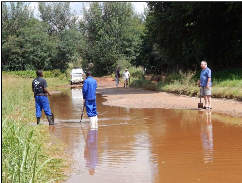
John Whillier (SCE127), and two of his workers, with, in the distance, Nic Rosenberg (SCE154) and Garfield Krige (SCE129) discussing the emergency plans to save the first bridge from collapsing
